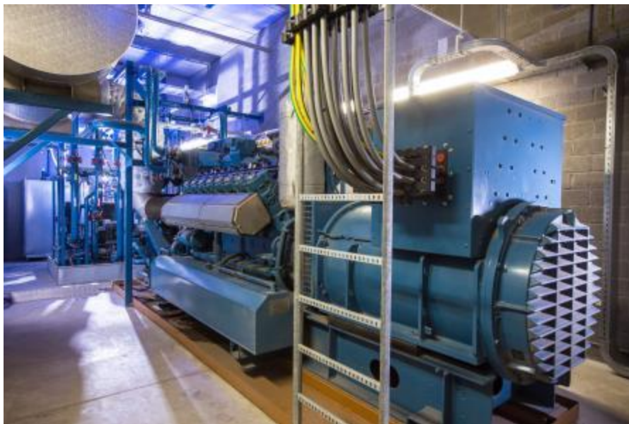
The first 1200 kW biogas engine (CHP unit)
