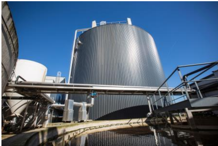
Remo-Frit plant featuring Global Water Engineering technology
