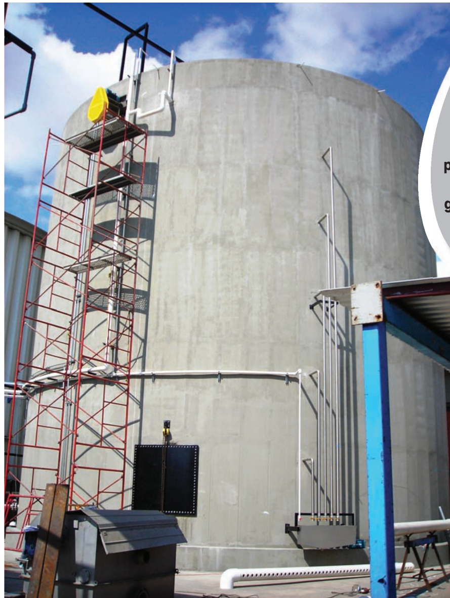
Figure 2: View of the Concrete ANAMIX™-T Reactor at the Final Stages of Construction.
