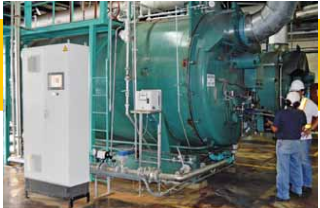
Ecuadorian brewery Cerveceria Nacional is introducing a second waste-to-biogas plant that expands on the success of its first plant, which already produces the equivalent of more than 6,000 kg of fossil fuel per day.
