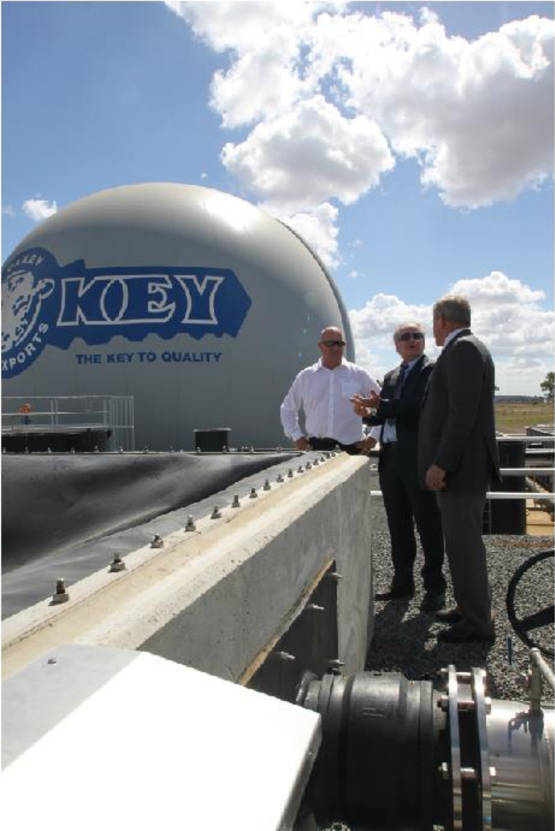
CST Wastewater Solutions Managing Director Mr Michael Bambridge, Centre, outlines the new Global Water Engineering plant to Minister Macfarlane, right, and NH Foods Mr Andrew Trianace
