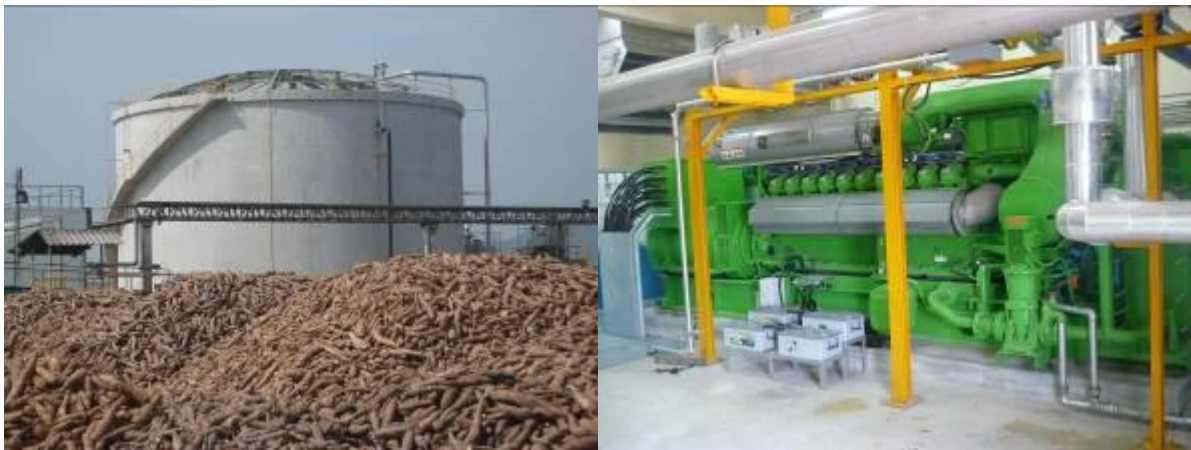
Chok Chai Starch plant with Cassava roots in the foreground, left and the generator, right
