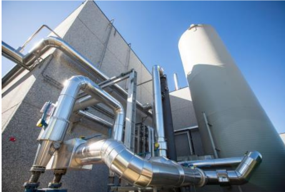
The BIOSULFURIX™ (right) and the GASODRIX™ (left) Biogas is first sweetened (BIOSULFURIX™) and dried (GASODRIX™) before it can be used as fuel for the biogas engine
