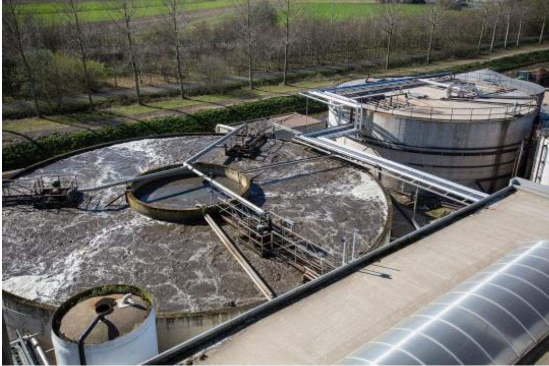
The wastewater treatment plant with the anaerobic reactor (ANUBIX™-B) at the right and the nitrification basin at the left
