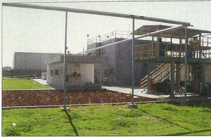
An anaerobic wastewater treatment plant (ANUBIX™-B) in a Frito Lay plant in Sabritas, Mexico produces 4,000 kg/day COD or 1,100 kg/day fuel oil equivalent. Photo by GWE
