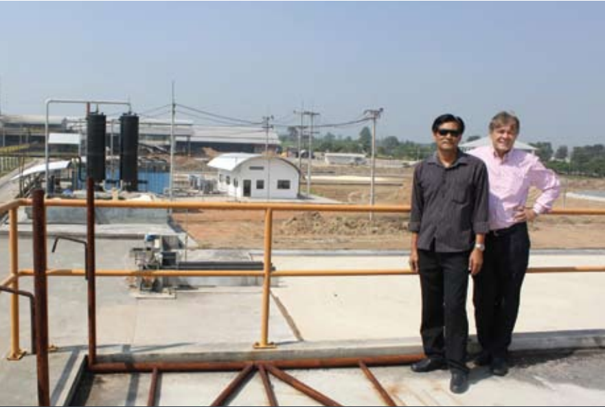
This shows the two scrubbers that are used to remove H 2 S (hydrogen sulphide) in the biogas before the biogas is sent to the gensets to make electricity.
