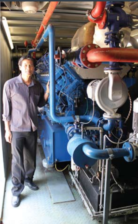
Tawatchai Yuenyong with the plant's generator sets that return power to the grid
