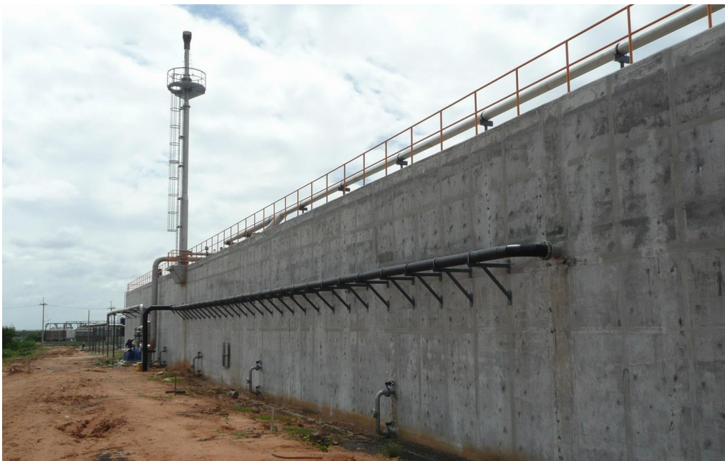
The reactor and biogas flare at Corn Products
