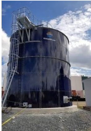
Organic Power Ltd. is installing a GWE Raptor anaerobic digestion plant in Bega Baja, Puerto Rico. Organic Power Ltd.
