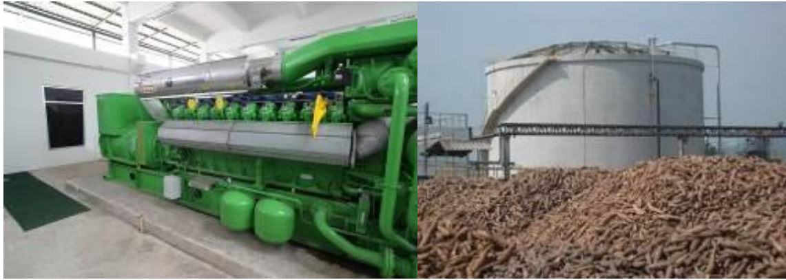
Green energy generators powered by biogas (methane) from waste water and wet pulp, transforming a problem to a profit. The Chok Chai project (right) won a global award for GWE
