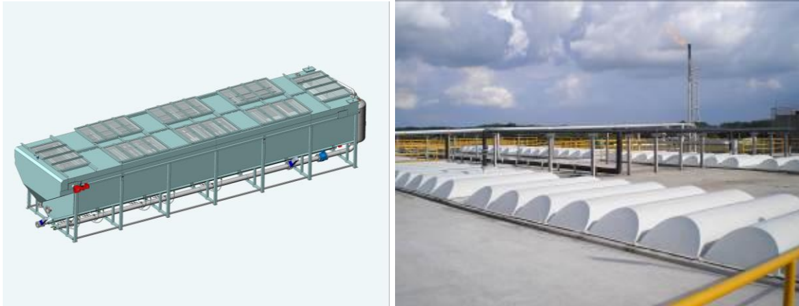
GWE technology deployed at the Cayuga dairy project in the USA, left, and the Vina Kraft paper plant in Vietnam. Cayuga features a completely enclosed SUPERFLOT-BIOGAS™ system for high efficiency removal of anaerobic biomass. Vina Kraft was a joint venture between the Siam Cement Group and the Japanese Regno Co Ltd, constructed to achieve world's best environmental standards
