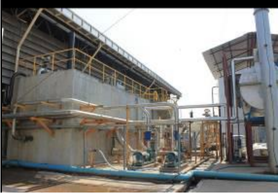
Pulp pretreatment and hot water boiler
