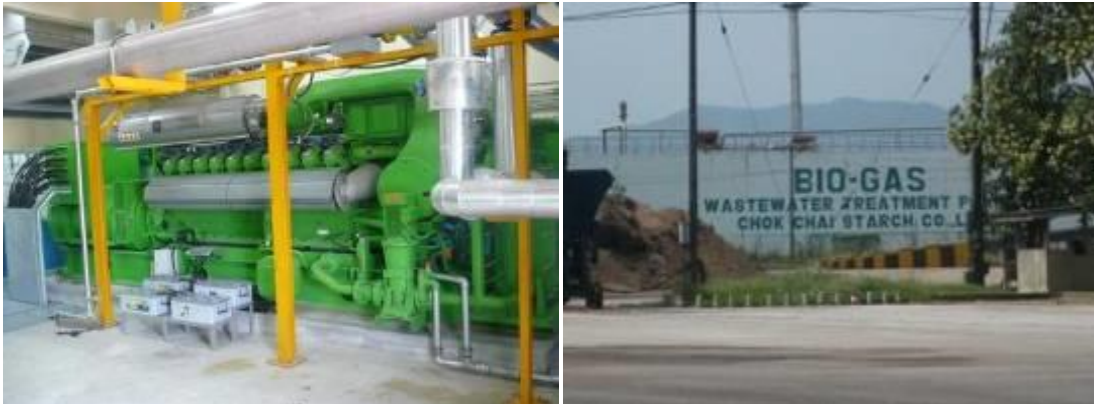
One of three Chok Chai Starch electricity generators Pre-existing ANUBIX™ B reactor, proven over 10 years
