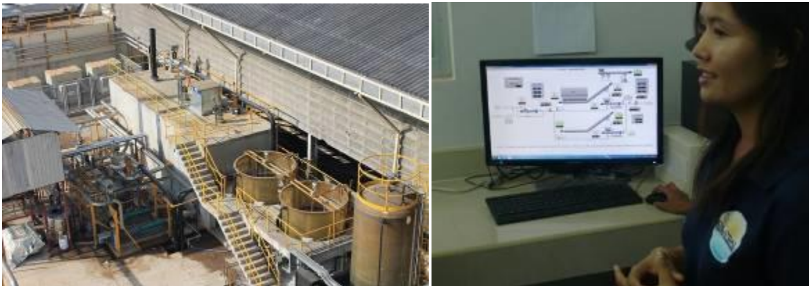
Pulp pre-treatment overview SCADA PC in the control room
