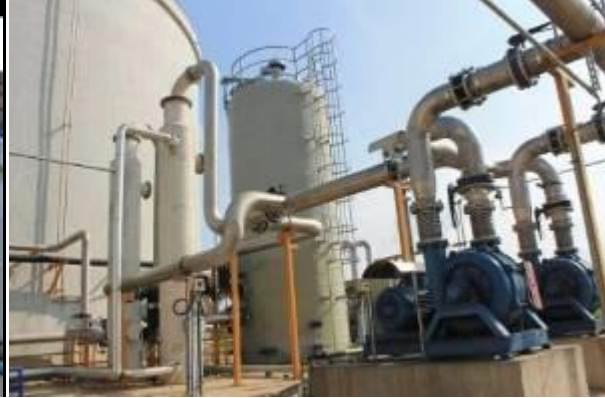
Biogas treatment and blowers
